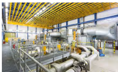
An example of a natural-gas compression station. (© Open Grid Europe GmbH)
