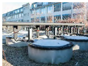
Ice storage at the Adlershof site. (copyright Anja Hanßke).
