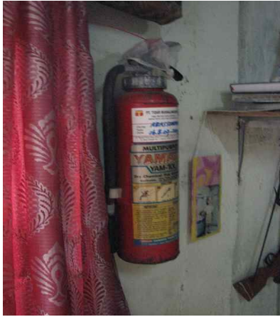
Fire Extinguisher in RT 10
