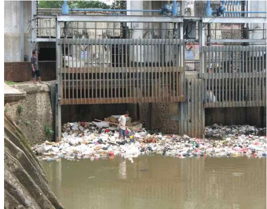
Clogged Flood Gate and Scavenger
