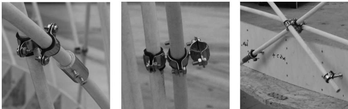
Figure 5-9: Aluminium tubes with contact hexagon sockets (left) were used to prolong the rods, double and triple (left, middle) swivelling pipe connections to connect the grid layers and single pipe clamps with screwed threaded pins to connect the rods to the edge timber ring
