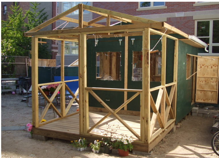
Figure 21, 22, 23: Prototype construction of the Gardenhaus at Vogue Community Garden at East 156th Street and Elton Avenue in the South Bronx, 2007. Photo: Carolin Mees.
