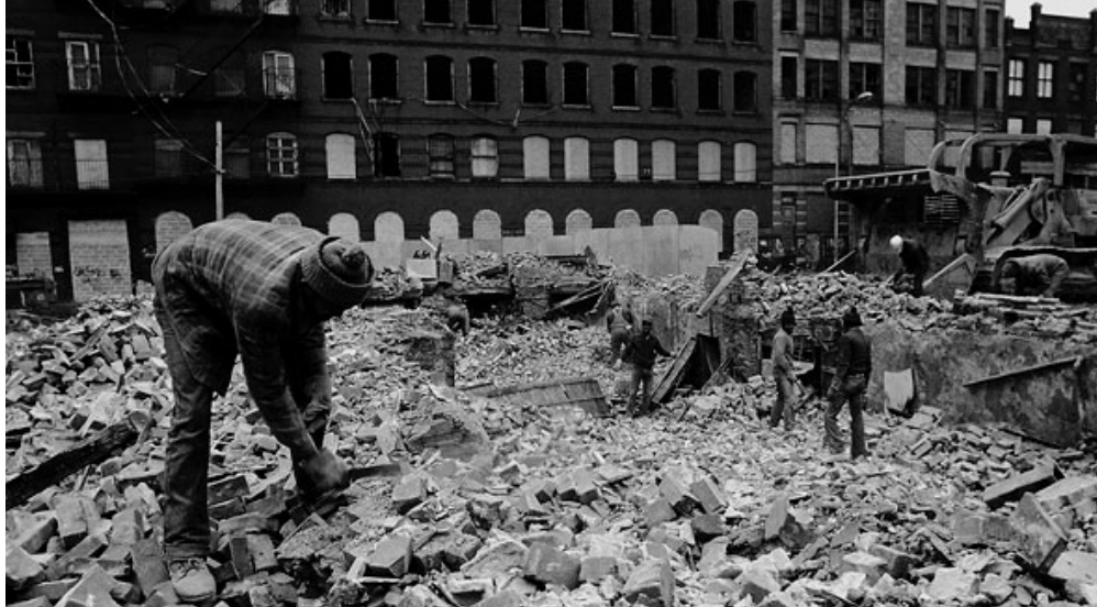
Figure 10: Rubble filled lot after demolition of an apartment building, 1983; © 2014 Lisa Kahane, NYC.
