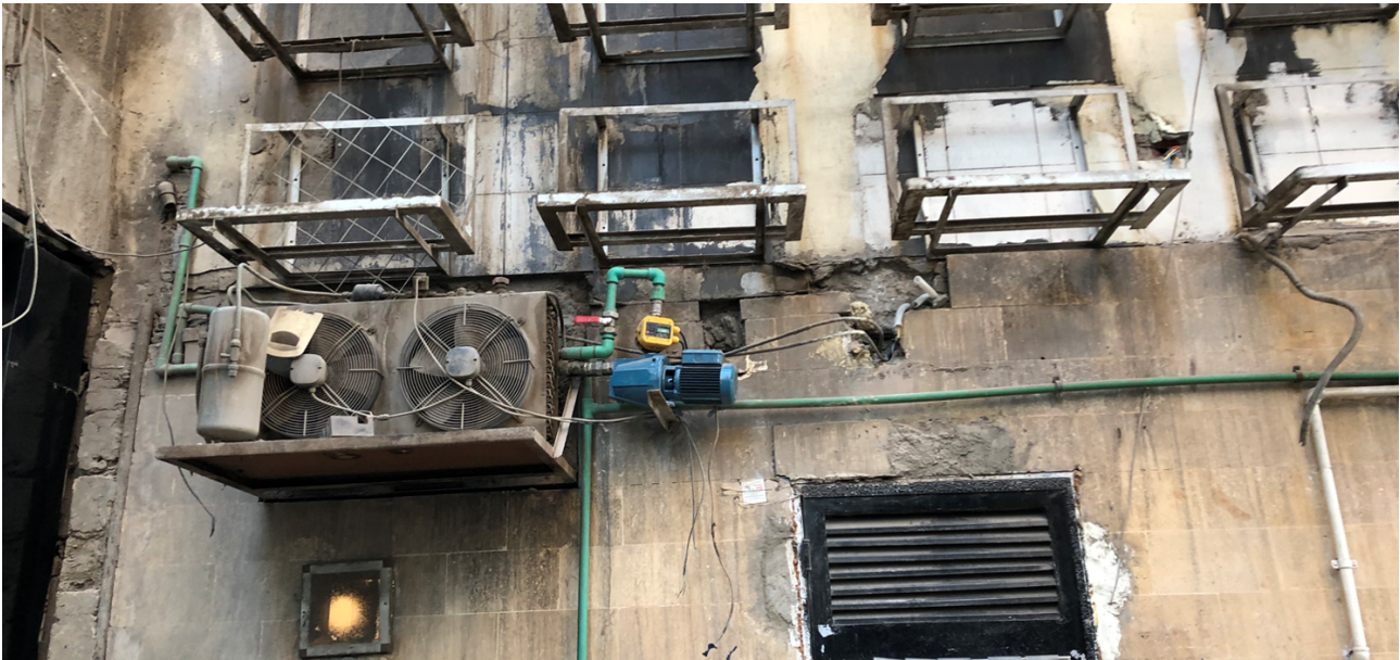
Figure 7.6.: Outdoor unit of a multi-split-unit at the road crossing of Ismail Mohamed and Yousif Kamel street on Zamalek, Cairo, Egypt, taken by the author on 10 November 2017.
