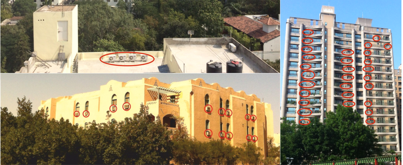
Figure 1.7.: Top left: Outdoor units of split-units on a rooftop in Hyderabad, India. Lower left: Packaged systems on an apartment building in El Gouna, Egypt. Right: Outdoor units on balconies of a residential building in Kaohsiung, Taiwan.
