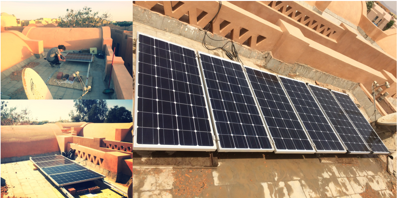
Figure 6.4.: Photovoltaic panels on apartment H12-214 during the erection (left side) and the final set-up on top of the apartment (right side).
