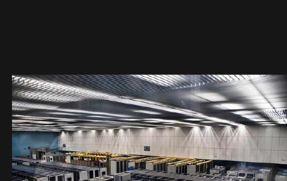
Server room in CERN. Photo: Florian Hirzinger, distributed under a CC-BY 3.0.
