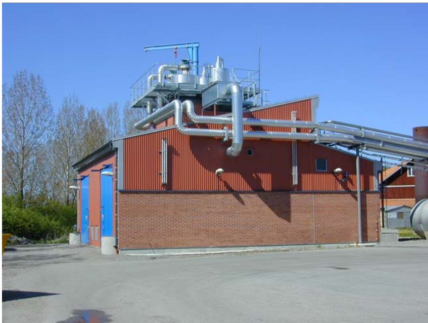
Fig. 6. The new upgrading plant.
