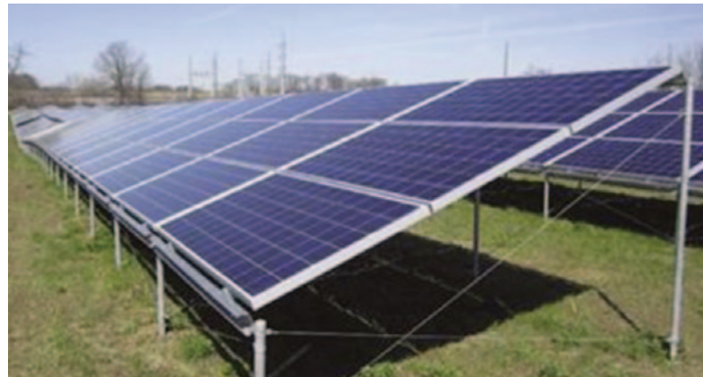
Figure 2: Structural system of photovoltaic structures affected by extreme wind actions.
