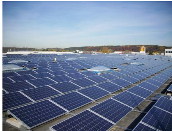
Abb. 5: Photovoltaik Dachanlage (online)
