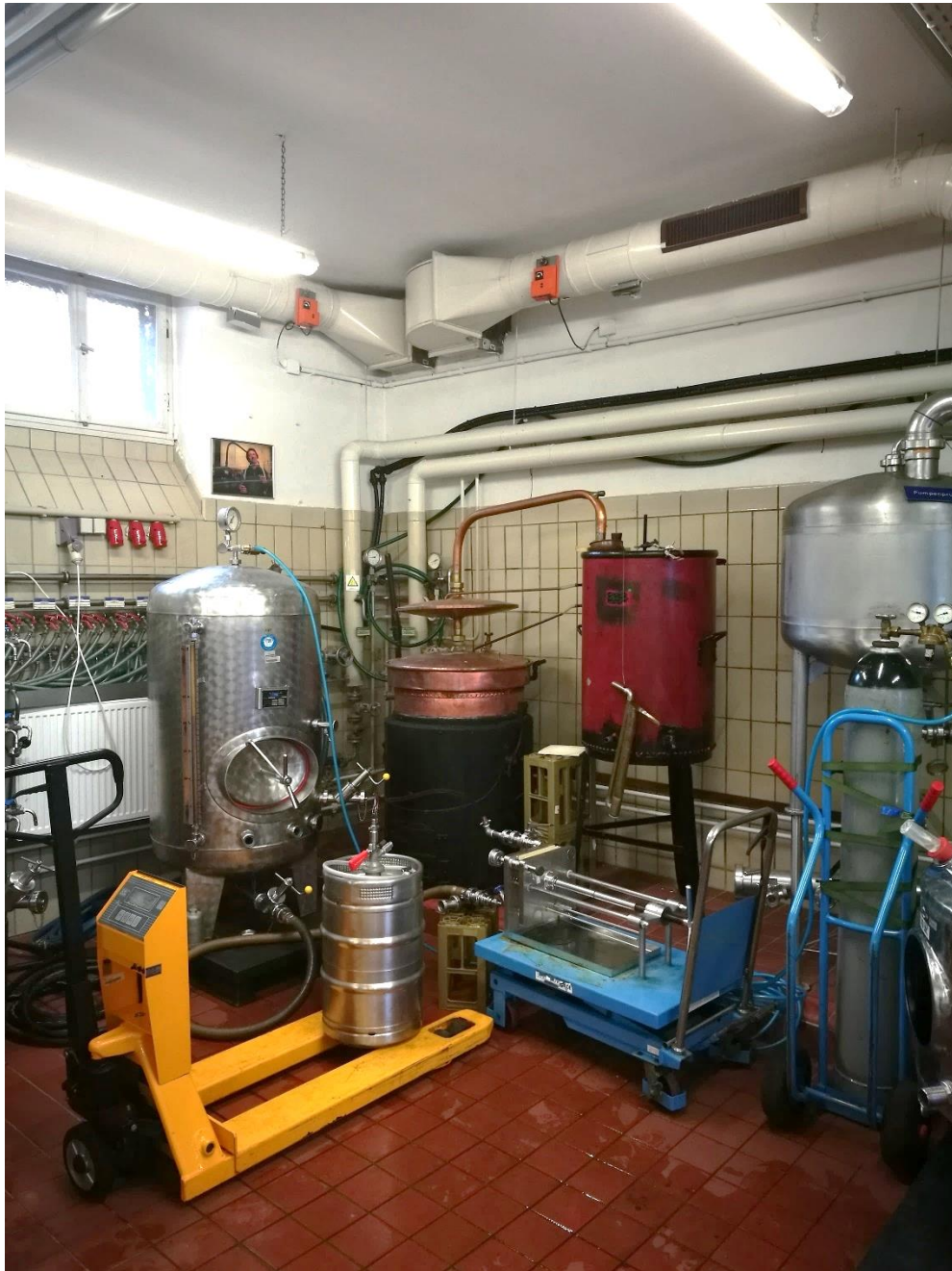
Figure 29. Wine filtration setup including pressurized stainless-steel tank, nitrogen gas tank, filtration device with plates, stainless steel keg for collecting filtrate and scale
