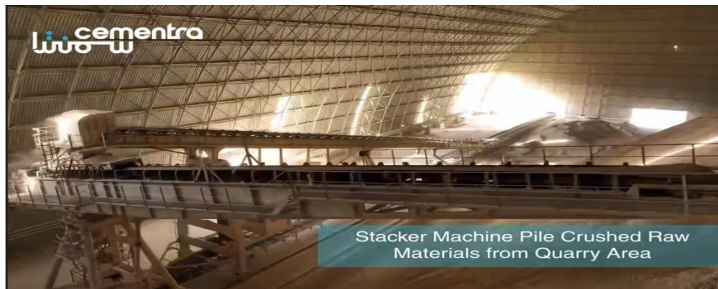
Figure 15, raw grinding plant, (cementra jordan, n.d.)
