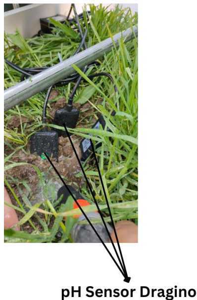
Figure 11. Photo of the soil pH sensors deployed in the test station.
