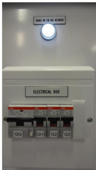
Fig. 6. Electrical part (Circuit breakers).
