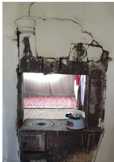
Stove placed between two walls used by 40% of household
