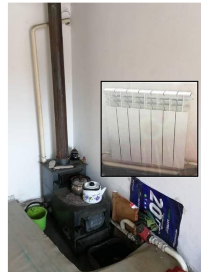
Stove with radiator heat distribution system used by 27% of household
