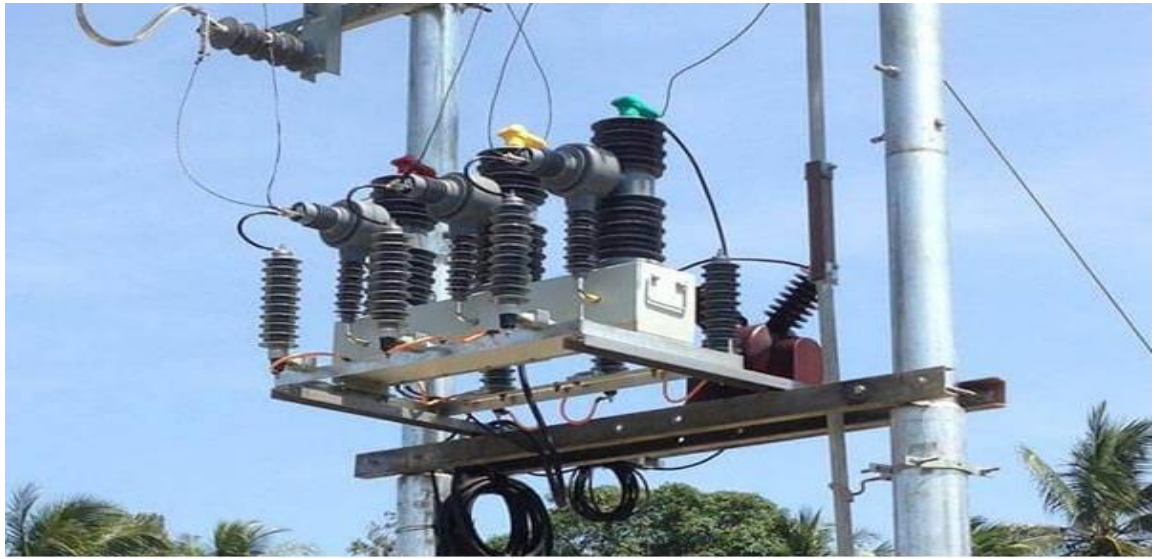
Figure 2. 5: Polemounted Recloser (Rockwill Electric Group, '2020)
