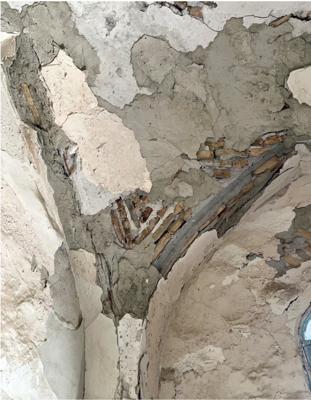
Scaling of different plaster layers in different stages, south-west corner
