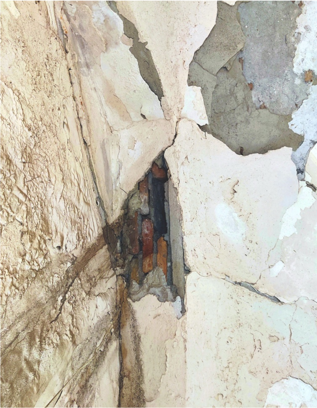
Water intrusion source in in northern corner of the cupola
