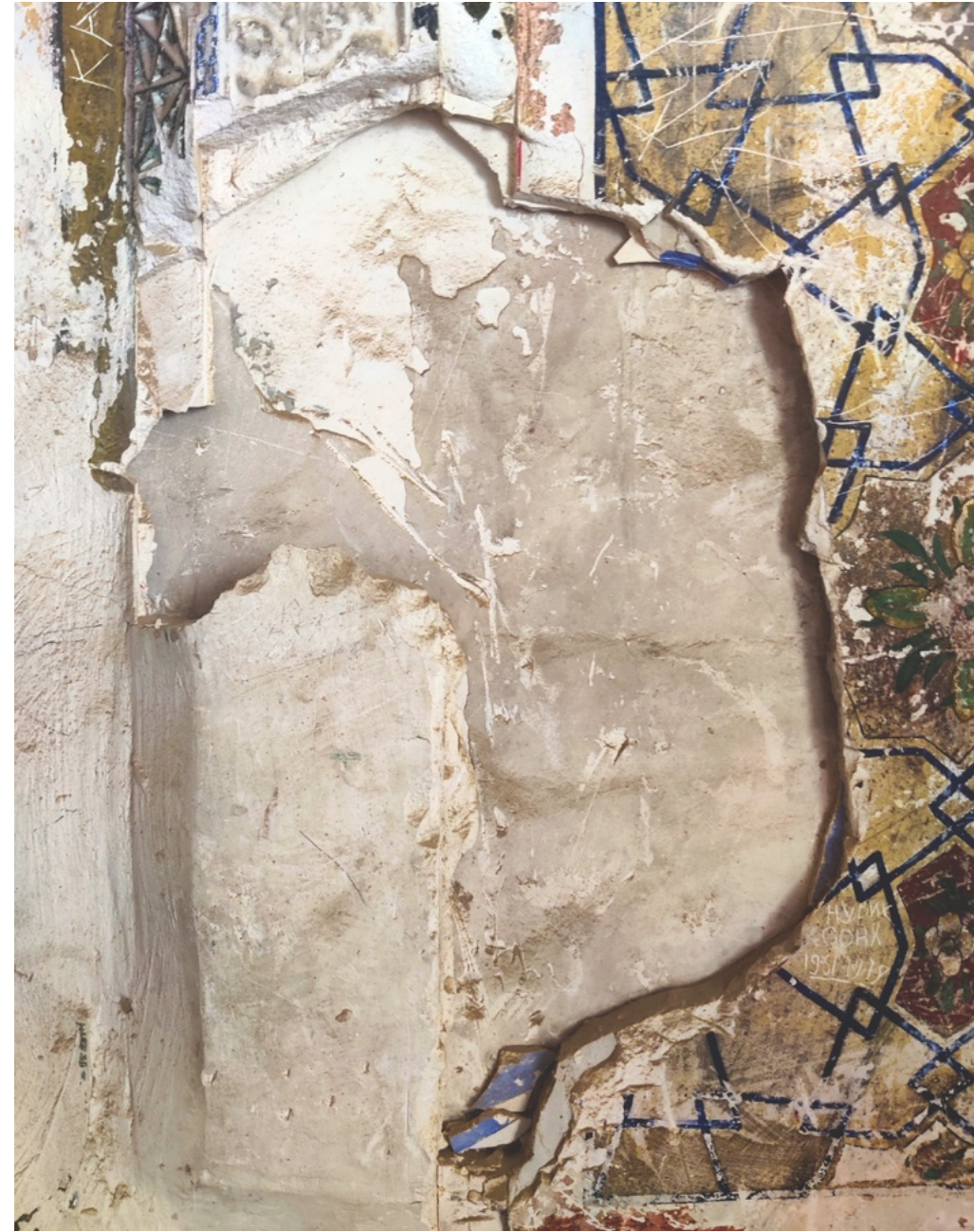
Loss of fragile wall paintings and stucco, south wall
