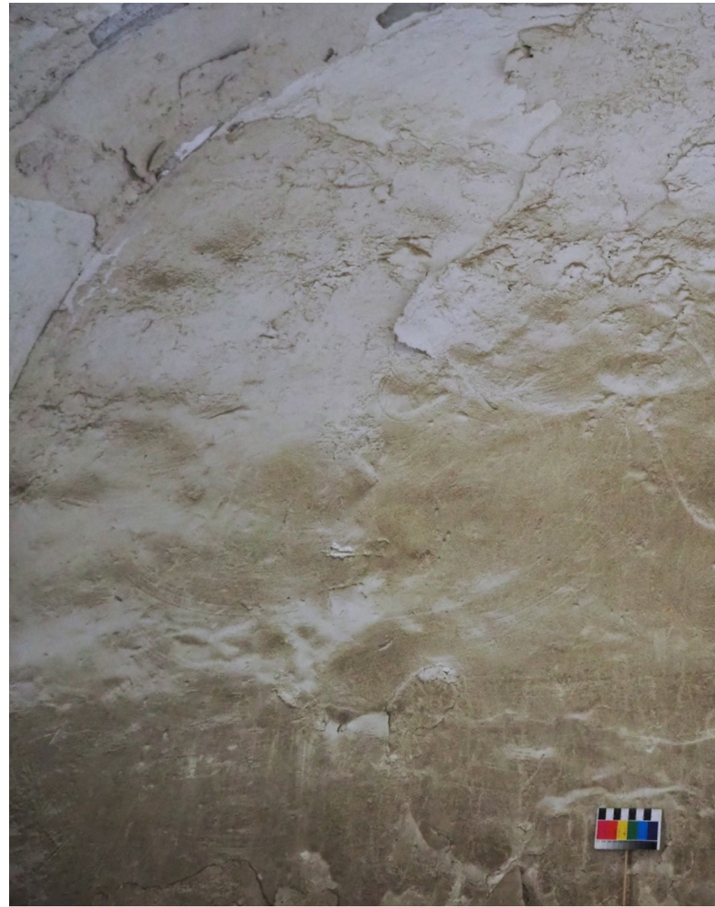
Crumbling of the upper plaster layer, north wall
