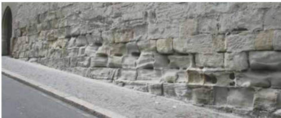
Figure 3: Lausanne (canton de Vaud, CH), rue de la Barre, Château Saint-Maire (10.04.2012). The sanding and disaggregation that affects the base of the building and up to 2 m in some areas is mainly due to the presence of NaCl.
