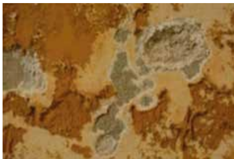
Photo 1: Deterioration of the inner walls due to salt crystallisation at Hagia Sophia, Istanbul, Turkey
