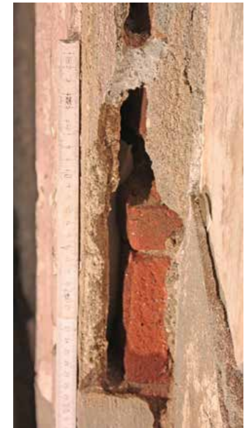
Figure 4: Delaminated pilaster in San Vincenzo Oratory, north wall
