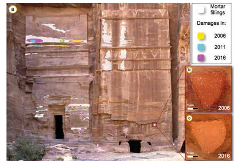
Figure 4: a) Ongoing damage progress of restored areas treated with silica-sol mortars during a period of 15 years on monument 825. b) Sample of a dry-slaked lime mortar just after application in 2006 and c) after 10 years.
