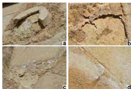
Figure 3: The damage forms on stone blocks. a) detachment of "artificial stone"; b) scaling and disaggregation of the original stone blocks; c-d) efflorescence on mortar joints and surface of artificial stone
