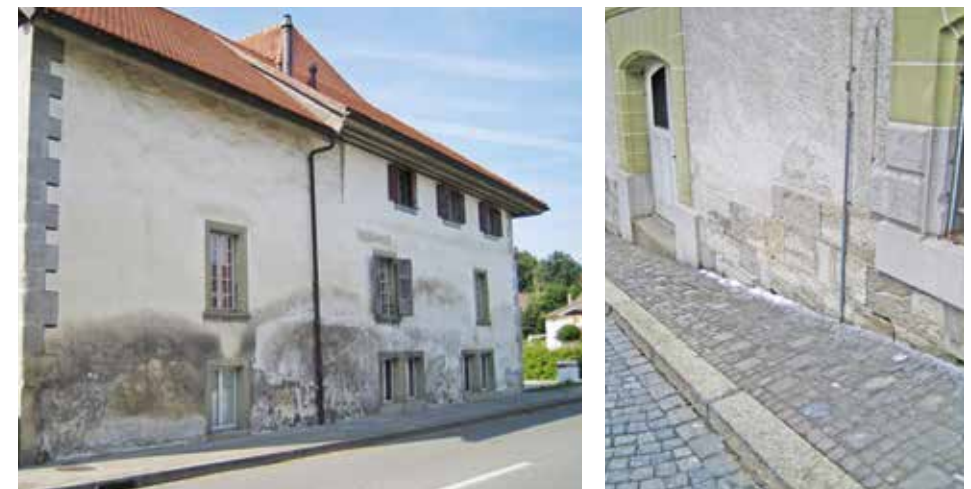
Figure 2: Left: Belfaux (canton de Fribourg, CH), north façade of the Lanthen-Heid manor (1526). The damages that affect the render and the underlying molasse-sandstone are mainly the result of splashing traffic along this street (3.09.2008). Right: Lausanne (canton de Vaud, CH), rue Saint-Etienne (20.01.2010). During dry winter cycles the residues of recrystallized deicing salts can be seen at the foot of façades that can either be mobilized and suspended in the air or enter the material when dissolved in water via hygroscopicity, rain, or more snow.
