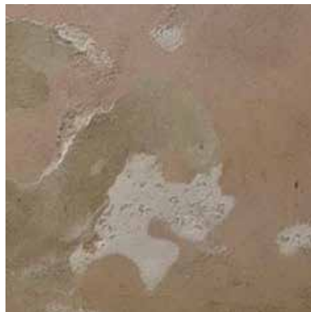
Figure 1: Overviews and details of salt efflorescences and moisture areas on granite and cement plaster covering the schist masonry
