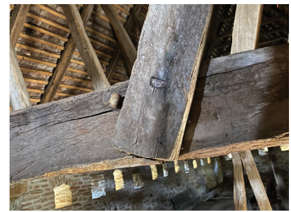
Fig. 3: Overleafing (distortion beam - corner strut) with metal nail.
