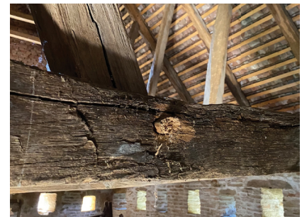
Fig. 4: Moisture damage to the distorted beam in the area of the connection with a corner strut.
