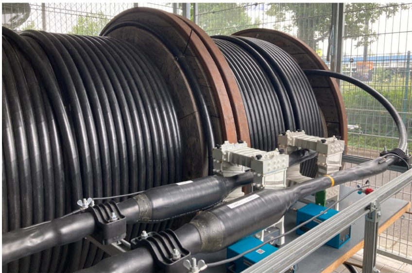
Fig. 7–6 Foreground: Joints with mounted HFCT prototypes and connected transient recorders. Background: MV cable drums. Published before in [Pub. 1].
