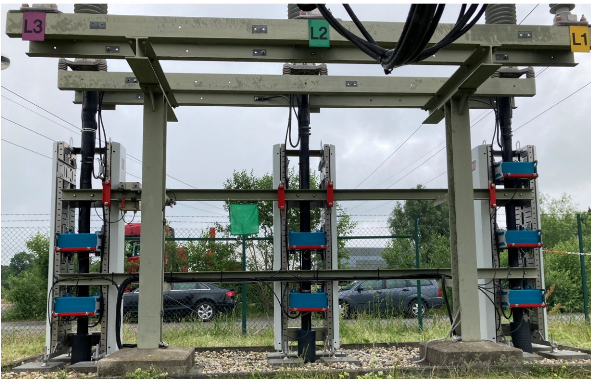
Fig. 8–1 HFCTs installed on the cable end terminations of 110 kV AC line.
