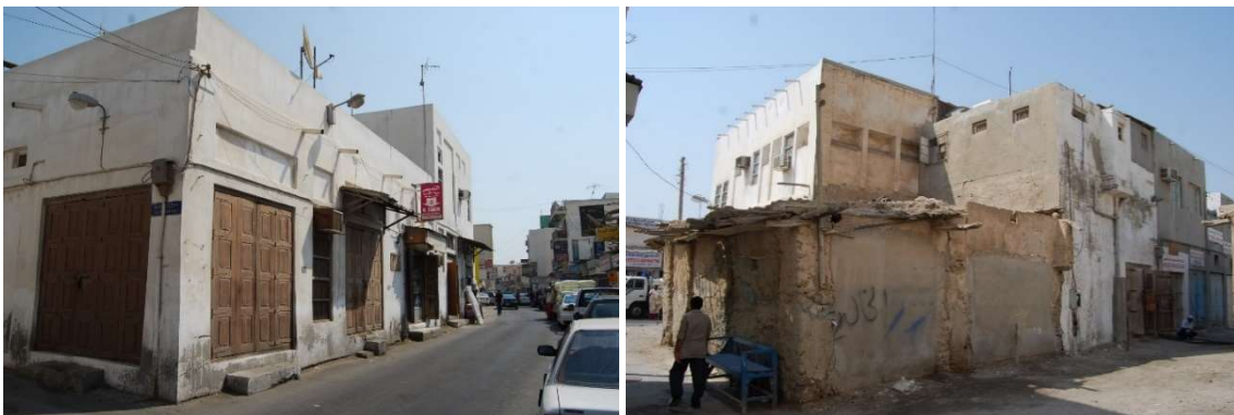
Fig. 3.4-7 and 3.4-8: The western Siyadi Shops on Tujjar Avenue and the one-storeyed shop units to their rear before rehabilitation in 2008. Photos: Eva Battis
