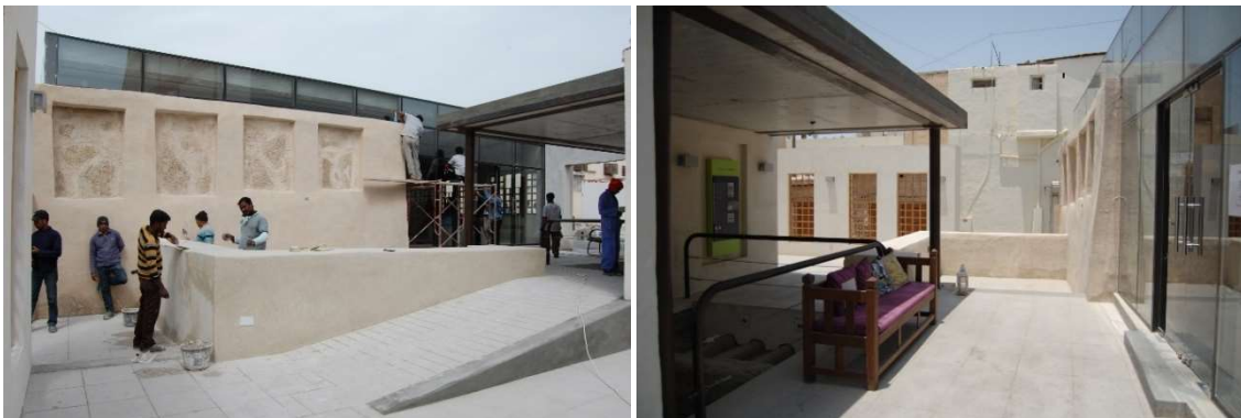
Fig. 3.4-25 and 3.4-26: The outdoor space of the eastern block during and after construction in 2012. Photos: Eva Battis
