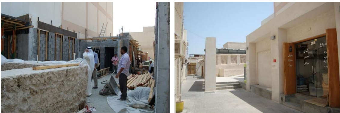
Fig. 3.4-27 and 3.4-28: The two shop units in the southern part of the site during and after construction in 2011 and 2012. Photos: Eva Battis
