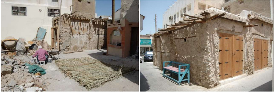
Fig. 3.4-19 and 3.4-20: The one-storeyed shop units to the rear of the western block during and after restoration in 2012. Photos: Eva Battis
