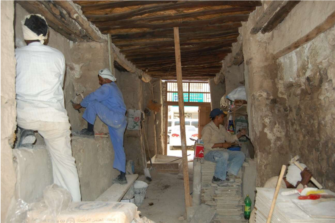
3.4.1 – 61: Removal of cement plaster inside the one-storeyed shops units of the western Siyadi Shops in 2012.
