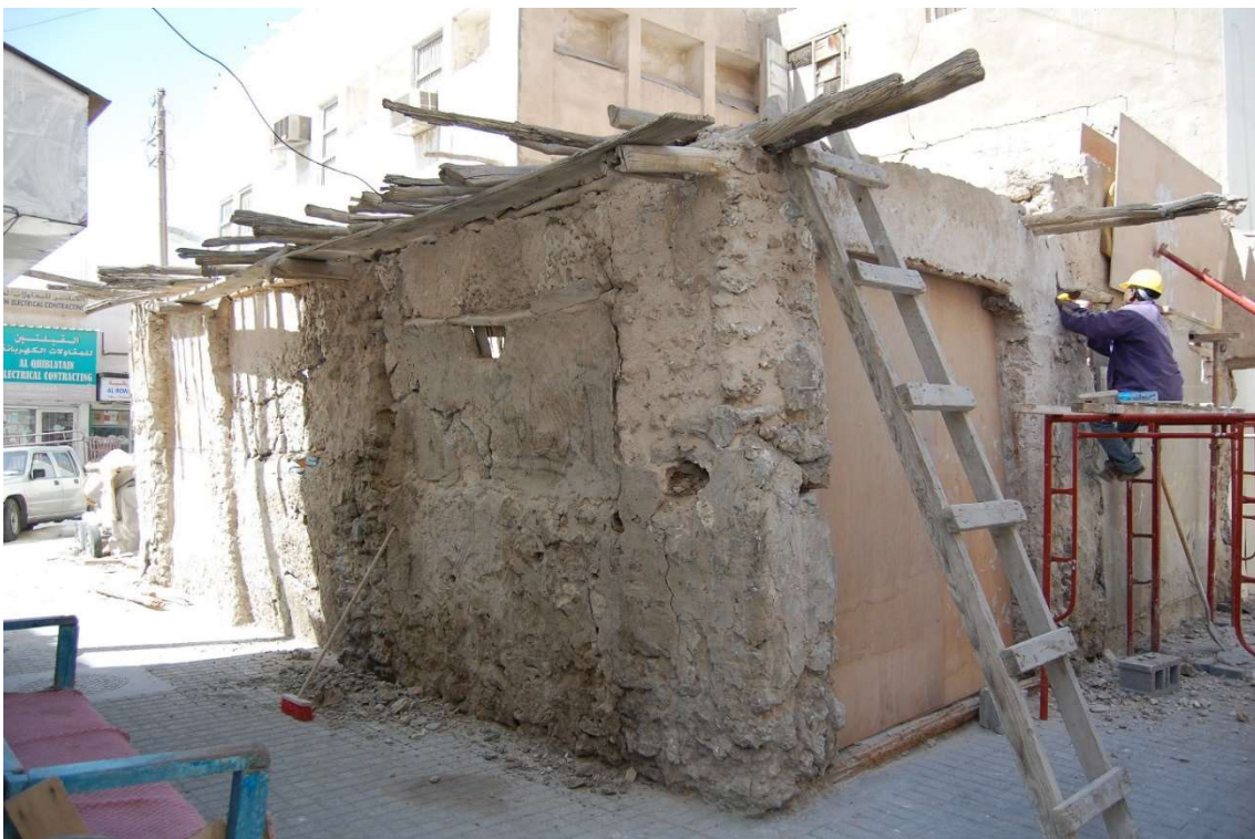
3.4.1 – 60: Chipping of cement plaster off the one-storeyed shops units of the western block in 2012.
