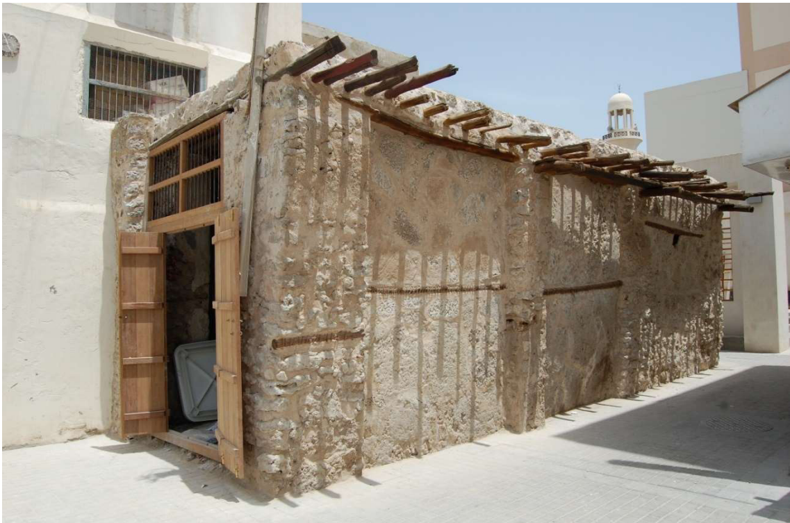
3.4.1 – 80: The one-storeyed units of the western block viewed from Tujjar Avenue in 2012.
