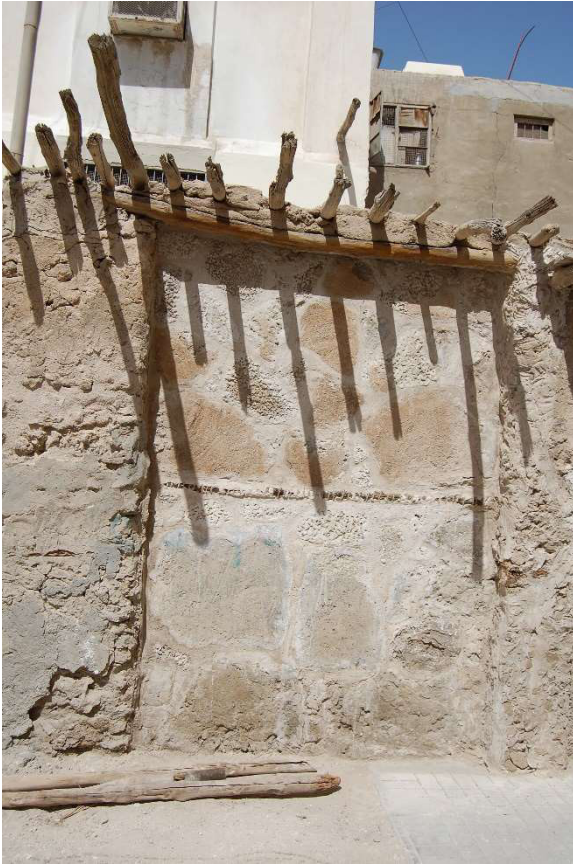
3.4.1 – 81: Repaired wall segment with coral stone slabs (farush) of the one-storeyed shops in 2012.
