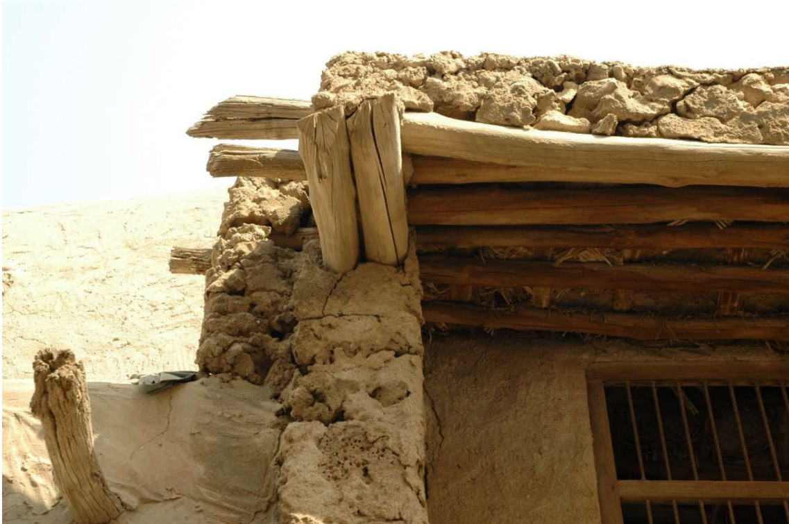
3.4.1 – 19: Western elevation detail of the ruined sixth unit of the eastern Siyadi Shops in 2008
