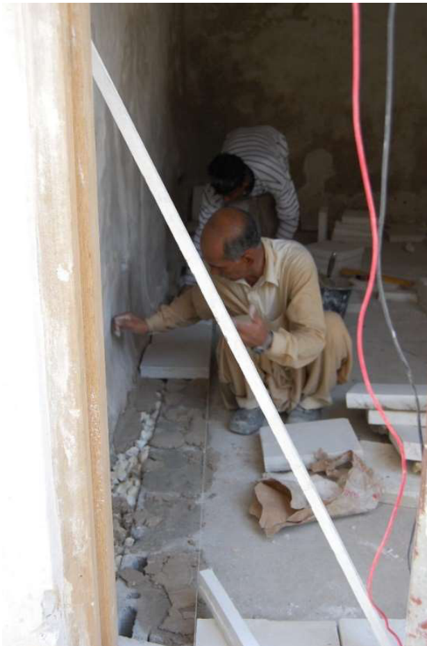
3.4.1 – 43: Construction of a ventilation trench in one of the shop eastern shop units in 2011. Photos: Eva Battis, Ministry of Culture and Information, Kingdom of Bahrain
