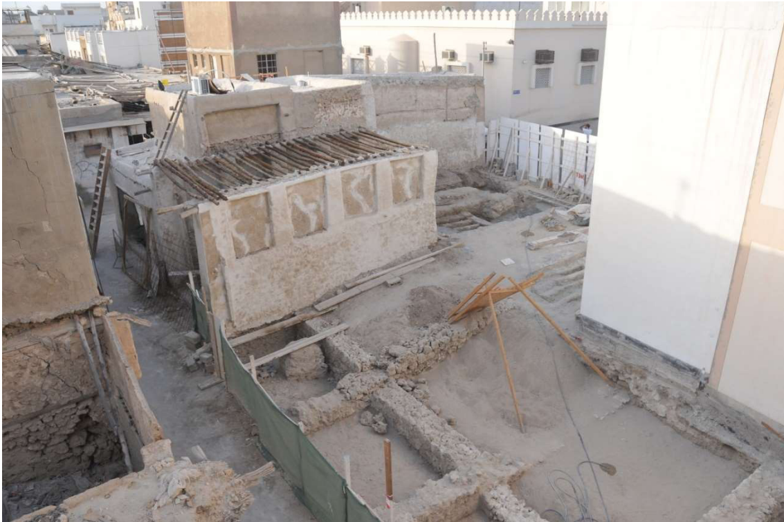
3.4.1 – 38: Bird's view of the eastern Siyadi Shops from the South-West during archaeological investigations in 2011. Photo: Dr. Alaa el-Habashi
