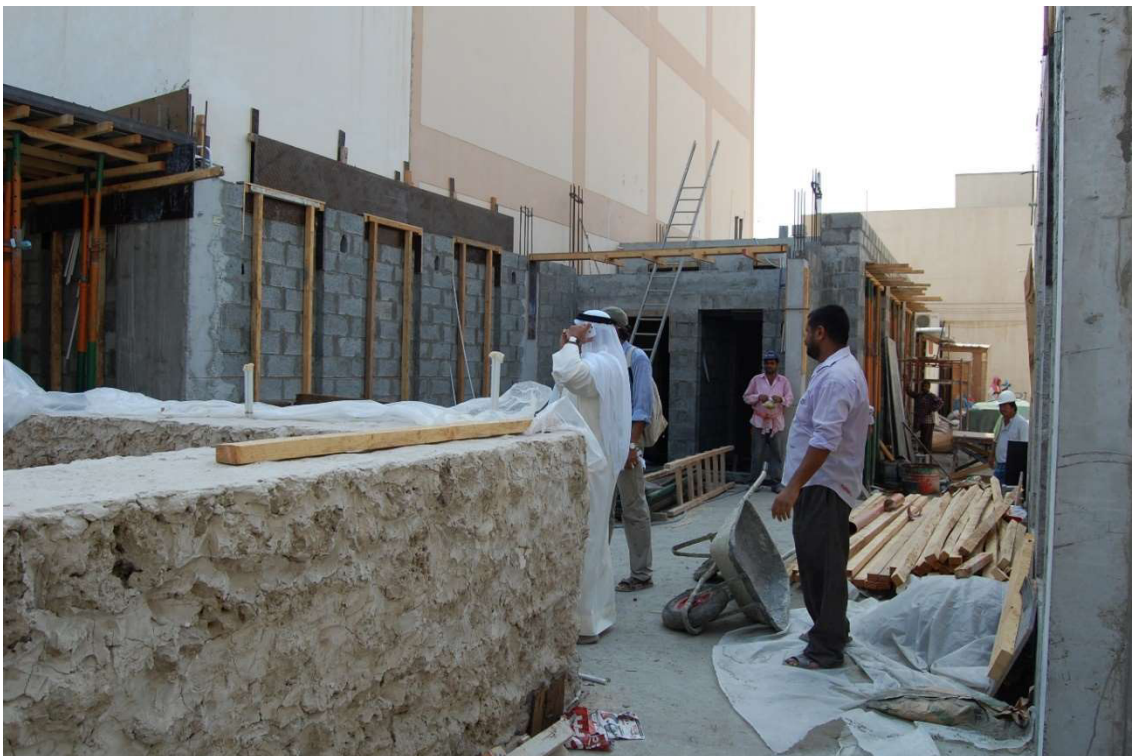
3.4.1 – 53: Additional southern shop units under construction in 2011 with reconstructed lower wall (left). Photos: Eva Battis, Ministry of Culture and Information, Kingdom of Bahrain
