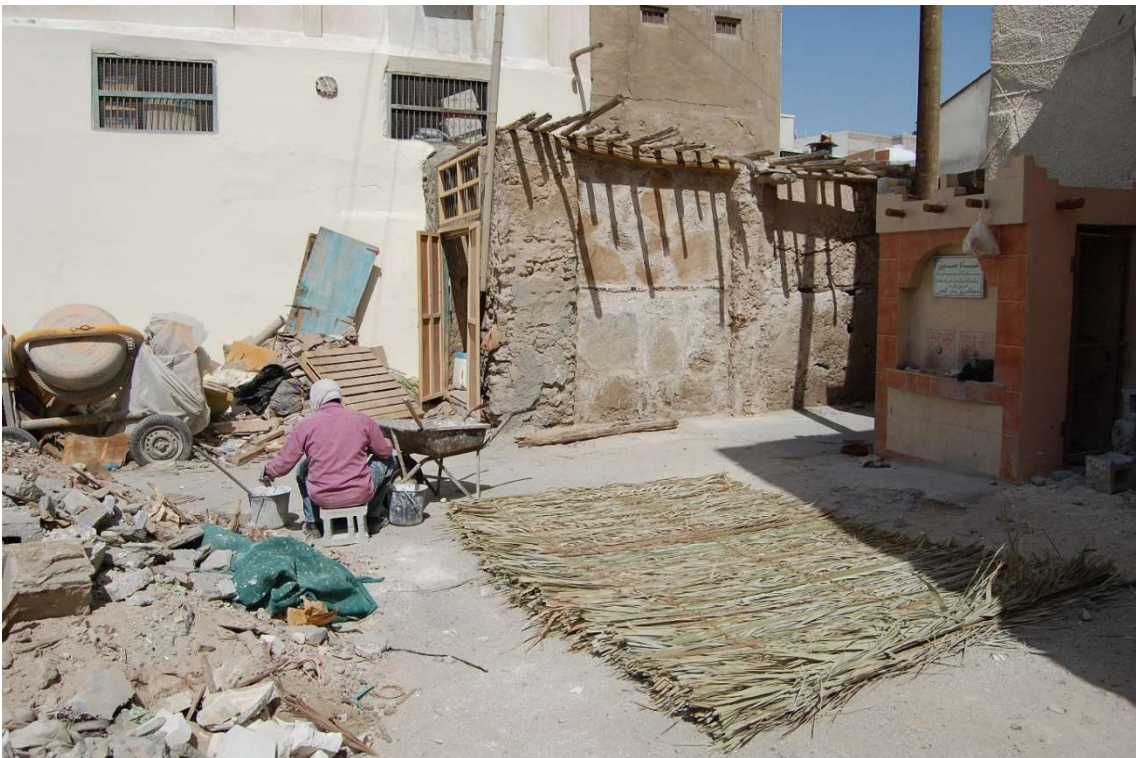
3.4.1 – 62: New palm frond ceiling mat before installation in the one-storeyed shops of the western Siyadi Shops in 2012.
