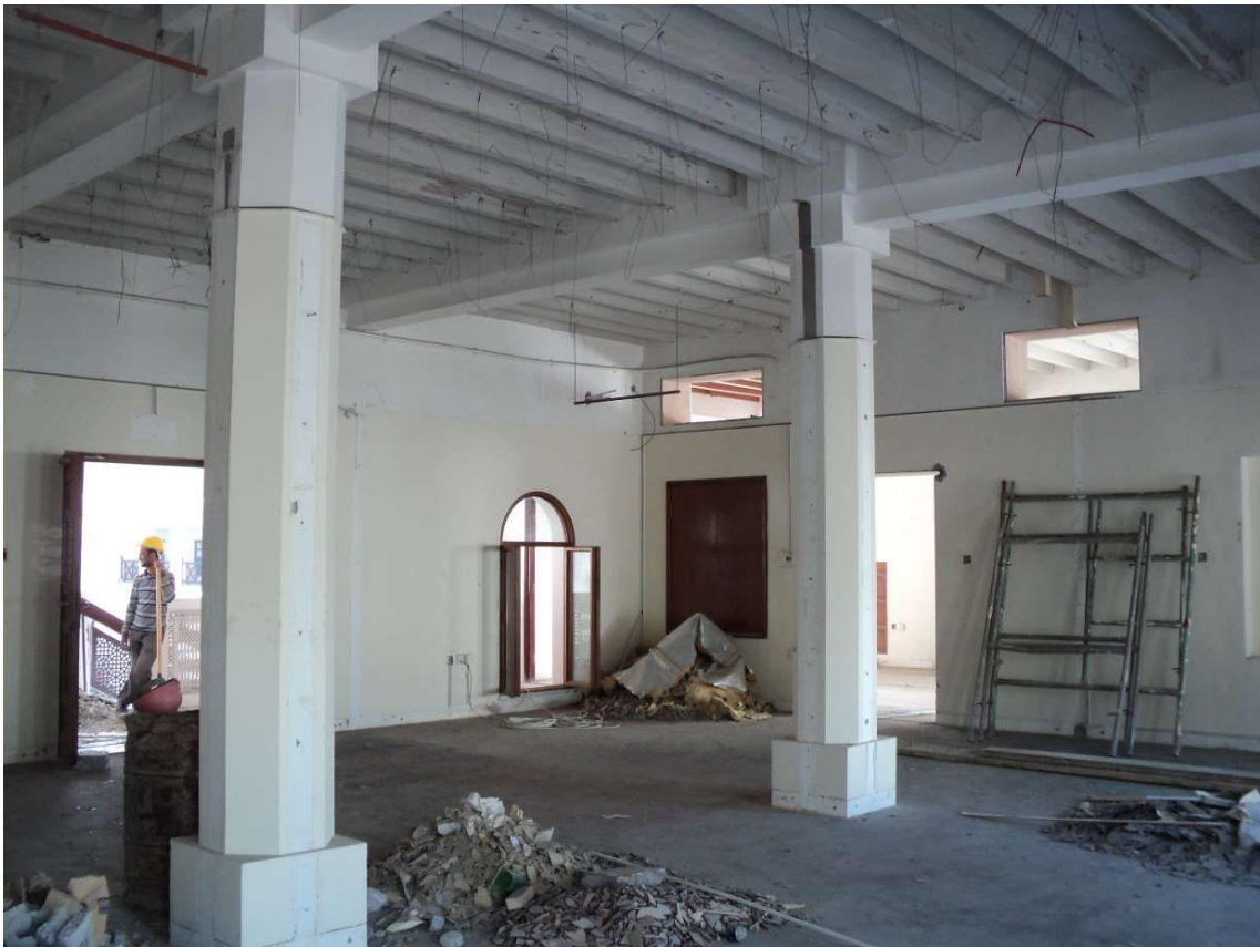
3.3.1 – 55: First floor hall during works and after removal of the suspended ceiling in 2012.
