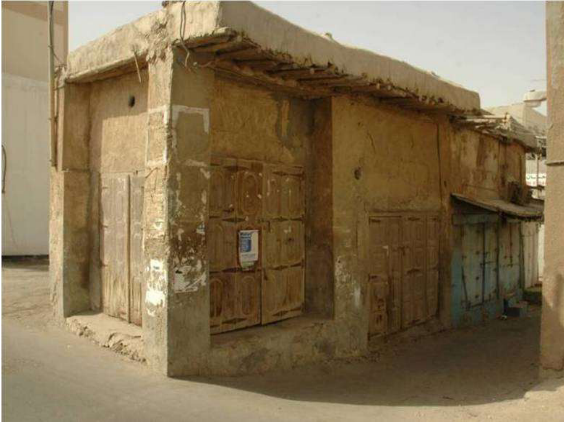
3.4.1 – 12: The eastern Siyadi Shops viewed from Bu Maher Avenue to the South-West in 2008 Photo: Dr. Alaa el-Habashi
