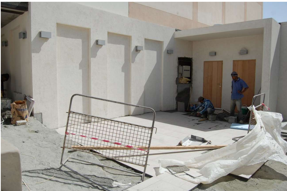
3.4.1 – 55: Outdoor space with sanitary facilities and new floor tiling being installed in 2012. Photo: Eva Battis, Ministry of Culture and Information, Kingdom of Bahrain
