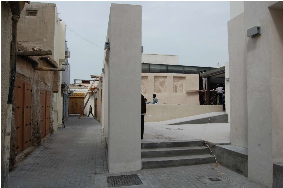
3.4.1 – 56: View to the North along the pedestrian lane and outdoor space during works in 2012.
