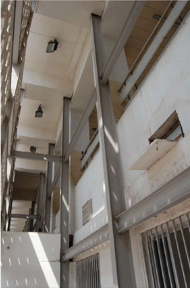
3.3.1 – 14: Detail view of the southern elevation with addition in 2014. Photo: Eva Battis
