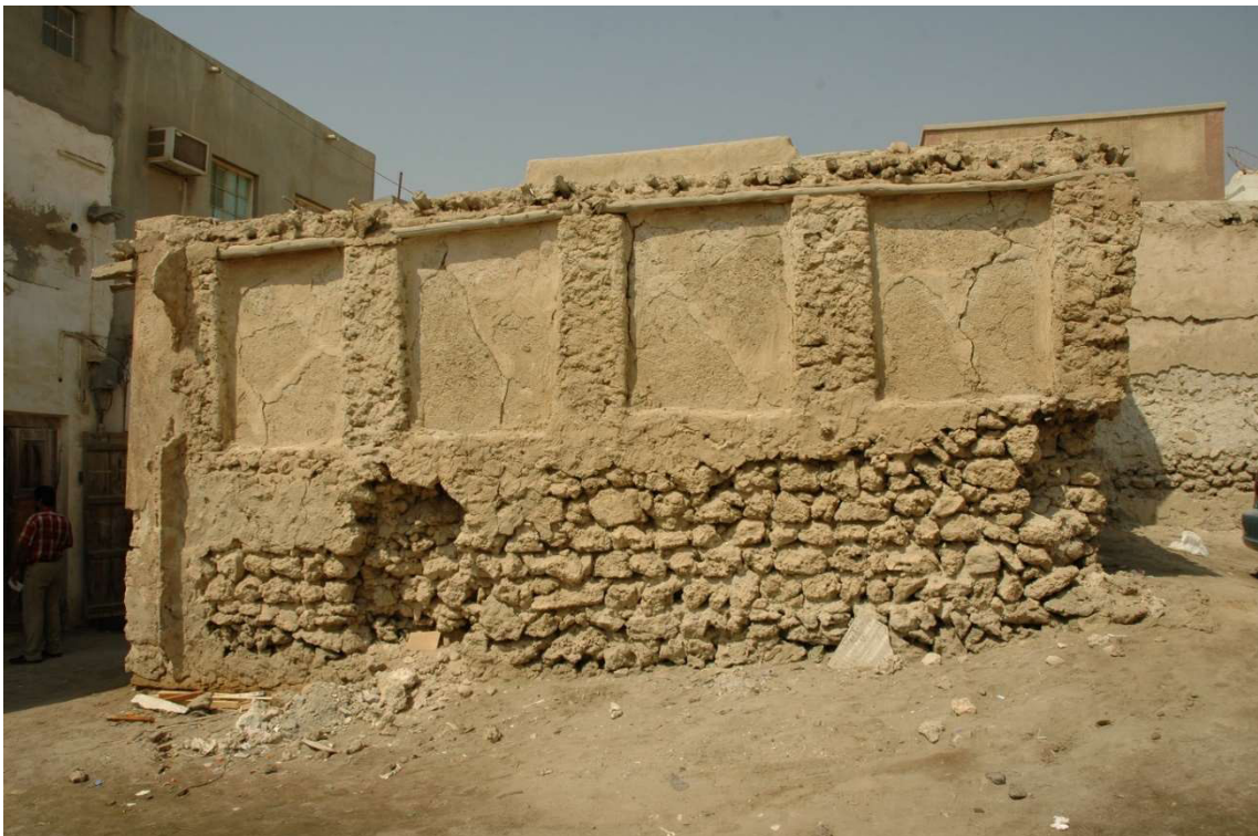
3.4.1 – 20: The ruined sixth shop of the eastern Siyadi Shops viewed from the south in 2008 Photos: Eva Battis, Ministry of Culture and Information, Kingdom of Bahrain
