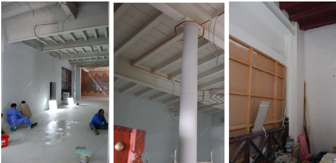
3.3.1 – 70, 71 and 72: View of the former post office premises and of the temporarily closed entrance loggia (right) during adaptation works in 2014.
