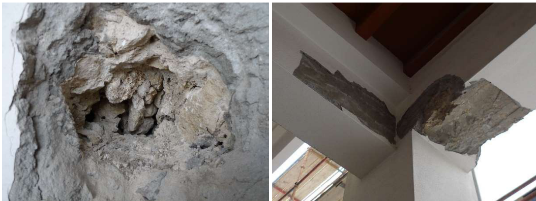
3.3.1 – 53 and 54: Details of wall structure and of ceiling joists from invasive investigations in 2011. Source photos: Plan Architecture & Design – PAD
