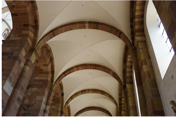
Fig. 8: Vault in the aisle of Speyer Cathedral, first half of eleventh century. The cross vaults on rectangular plan are designed with defined curves over the groins, like in Gothic vaults.
