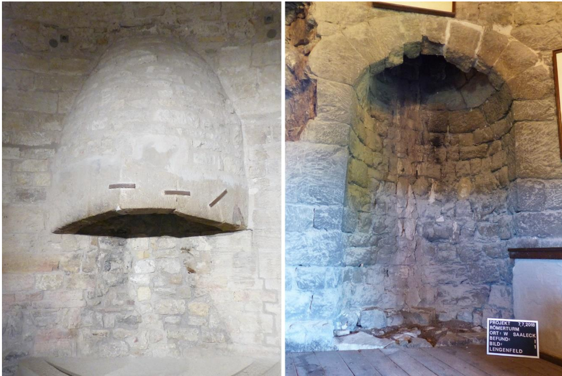
Fig. 13. The chimneys in Bergfried III of Neuenburg castle (1180) and the tower of Saaleck castle (1200) (left to right). (author)
