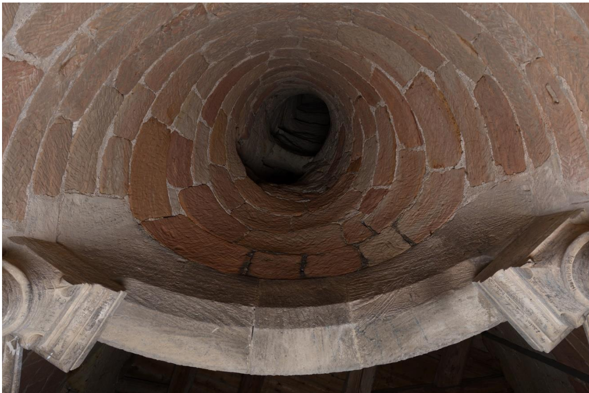
Fig. 8. View up the chimney flue from the fire room. Note the highly complex geometry and the second channel. (R. Wieczorek)
