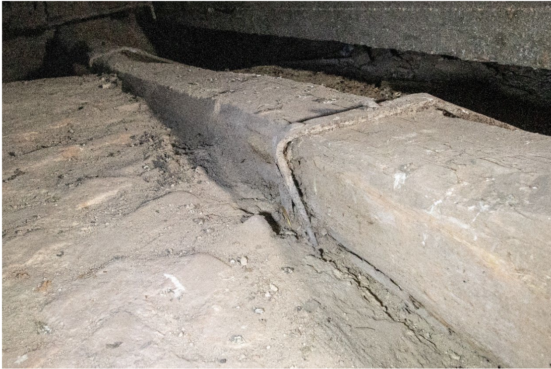
Fig. 10: Two iron bands attaching the double-curved arch above the organ gallery to a wooden beam.
