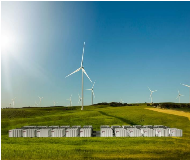
Figure 6 – Tesla Battery Power System in Jamestown, South Australia [19]
