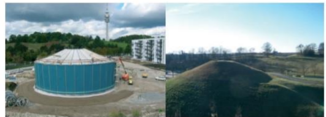
Figure 5 –Large Hot Water Storage (construction and final state) combined with Solar Thermal District Heating “Am Ackermann-bogen” in Munich, Germany [17]
