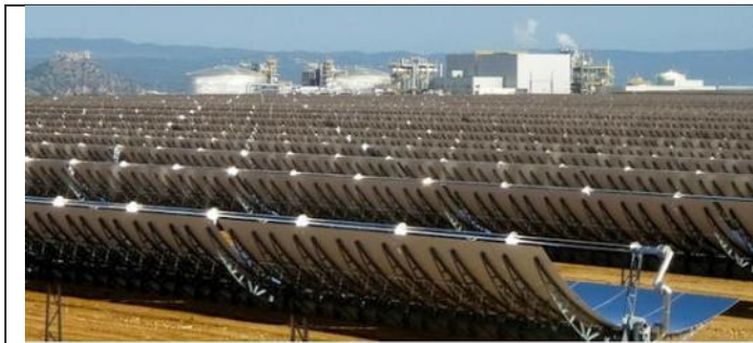
Fig. 7: Solar thermal power plant Noor 1 in Morocco
