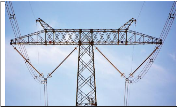
Fig. 15: Power pole of a HVDC system with 800 kV [11]
