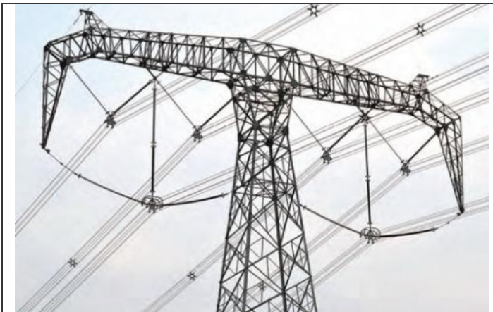
Fig.11: Power pole of a HVAC system with 1.000 kV [12]
