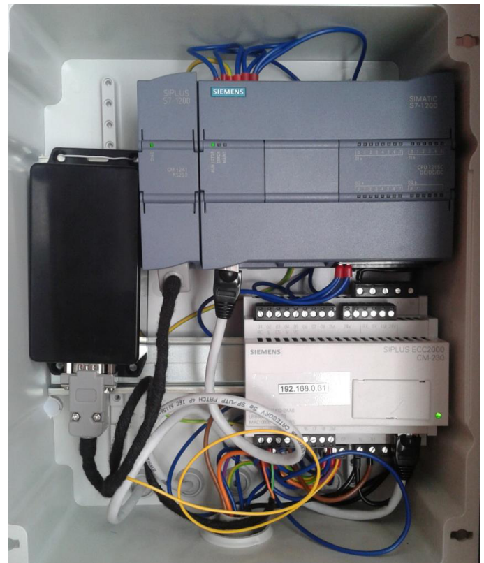
Figure 1. Devices in charging station
