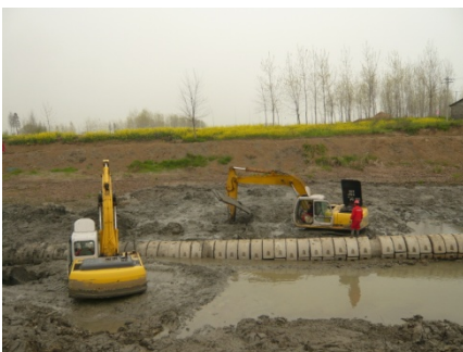
Figure 6: Adding heavy stuff onto gas pipelines
