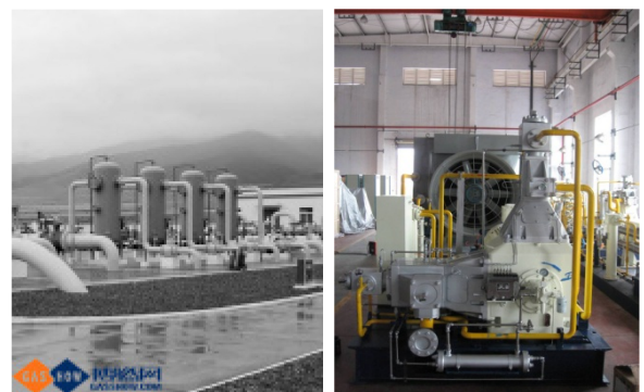
Figure 4: Hudong natural gas compressing station and compressor [7]
