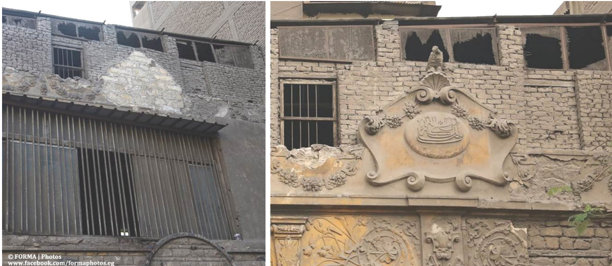
Fig. 3.1: The right photo (2013) shows decorative features that were deliberately removed as shown in the left photo (2019) in fear of official registration of the building in Cairo
