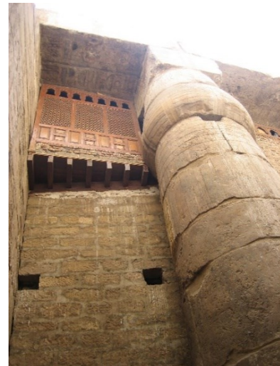
Fig 5.15: An opening in Abu Al-hajjaj Mosque (located in figure 5.17) incorporated in the structure of Luxor Temple Source: Khamis 2012a
