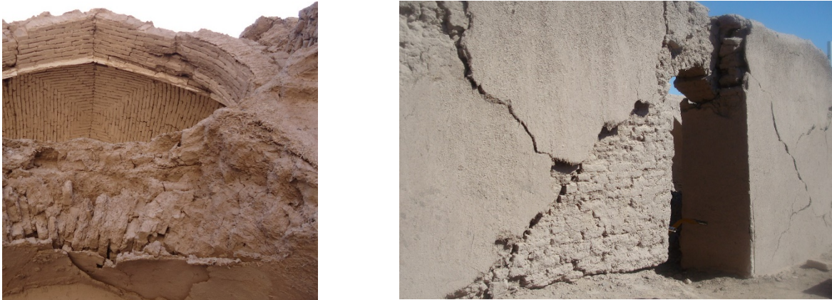
Figure 2-12 left: Sun-dried mud bricks (Khesht) in a collapsed adobe roof (Author, 2013), right: Earthquake-induced cracks on an adobe wall made of Khesht and Chineh (author, 2008)
