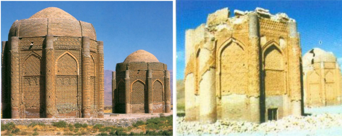
Figure 2-5 left: Kharraqan Tomb Towers before the earthquakes 2002 (ICHHTO), right: Collapse of the tower's dome (Hazrati 2003)
