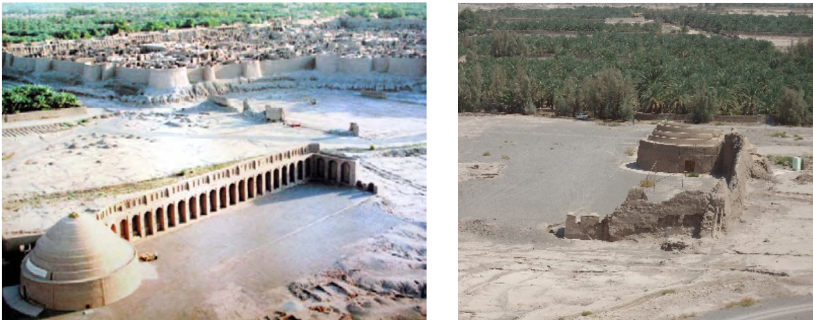
Figure 5-13 left : Icehouse before the earthquake (ICHO, 2004), right : Icehouse after the earthquake (Author, 2013)
