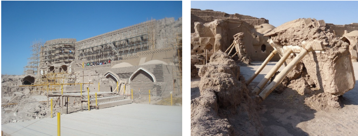
Figure 2-13 left: Post-disaster restoration of the Governor's quarter and the wooden visitor passage (Author, 2008), right: Post-earthquake stabilization of collapsed walls (Author, 2013)
