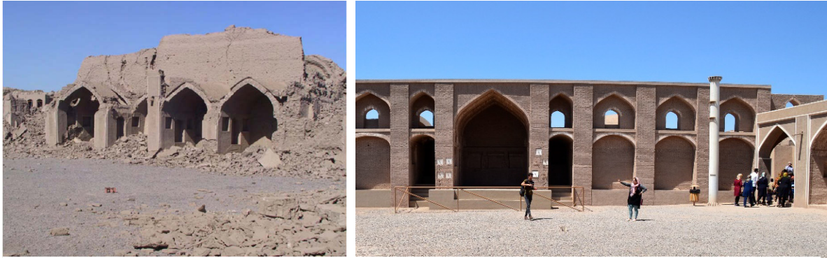
Figure 5-10 left: Tekiyeh after the earthquake (ICHO, 2004), right: Tekiyeh after the post-earthquake restoration (Felicitas Ernst, 2018, taken for the author)
