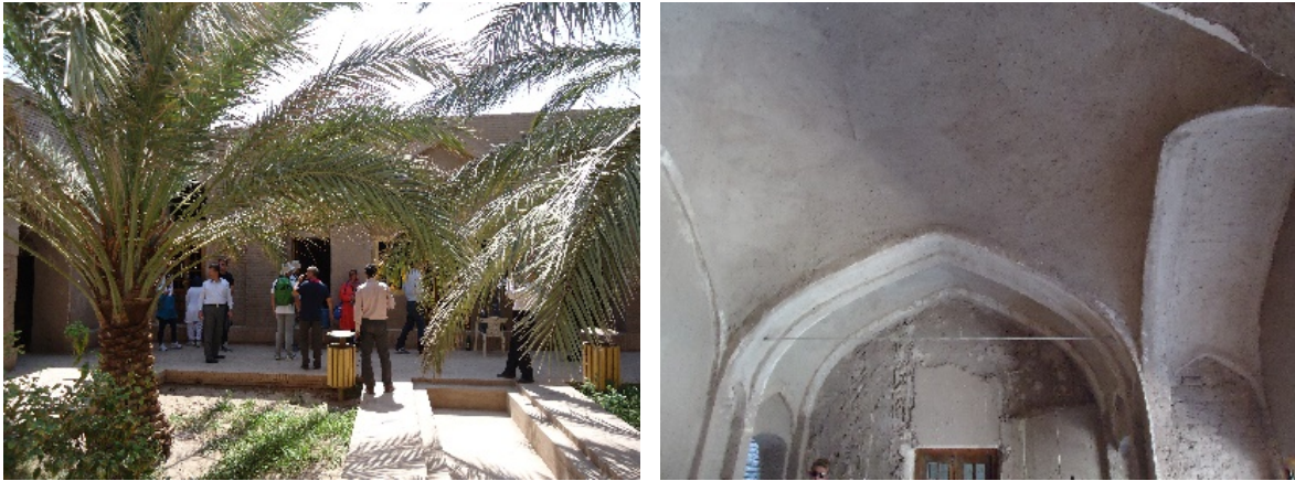
Figure 5-8 left : Sistani house after the post-earthquake restoration (Author 2013), right : The post-earthquake reinforcement in Sistani house (Author 2013)
