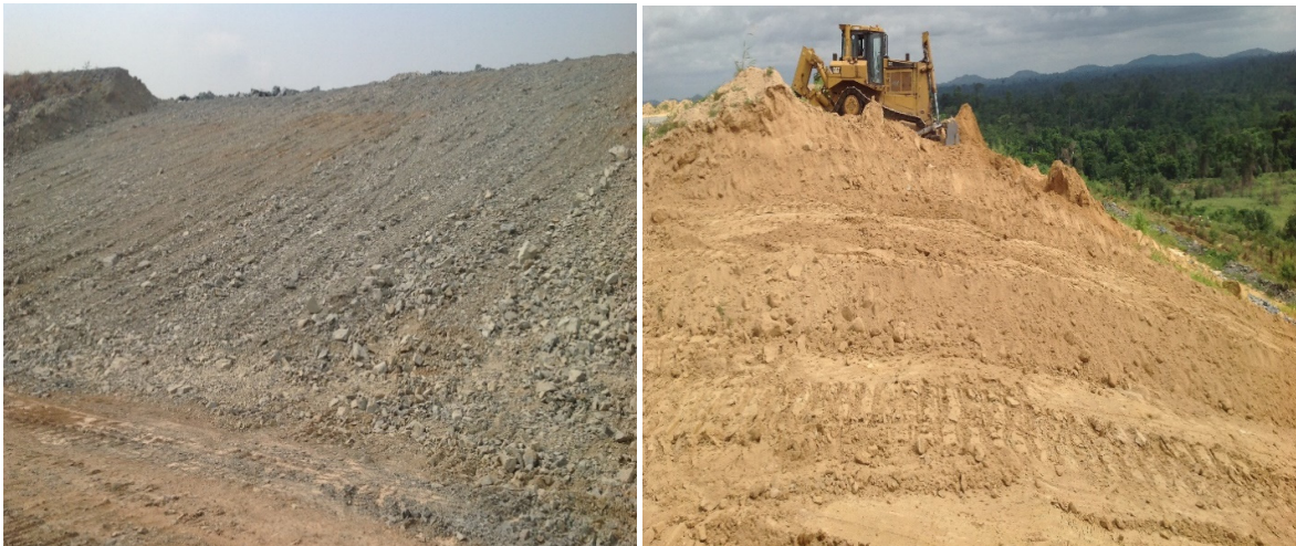
Figure 4. 2: The graded waste-rock dump (left); replacement of the STS on the graded rocks (right).
