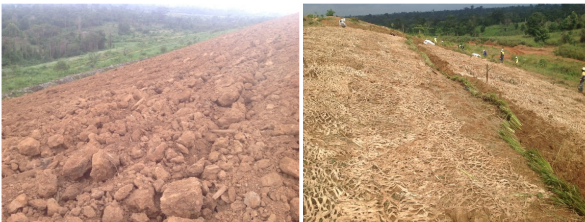
Figure 3. 3: Scarification after STP re-instatement (left), BGTs installation and vegetative planting of Vetiver grass stalks (right).
