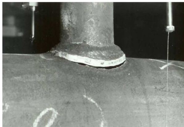
Figure 2.7: Weld failure in Vierendeel truss, T-joint CHS [52].
