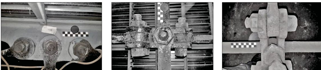
Figure 1.7 – Details of bearings and connections for the case–study of iron roof trusses in the State Hermitage Museum in Saint Petersburg [BTU CS (2011)].
