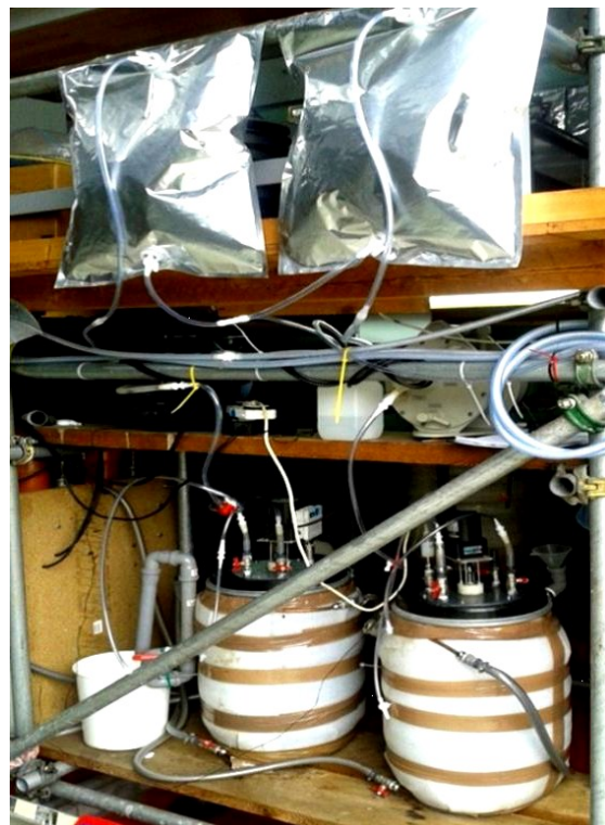
CSTR-rear view with biogas filled sacks
