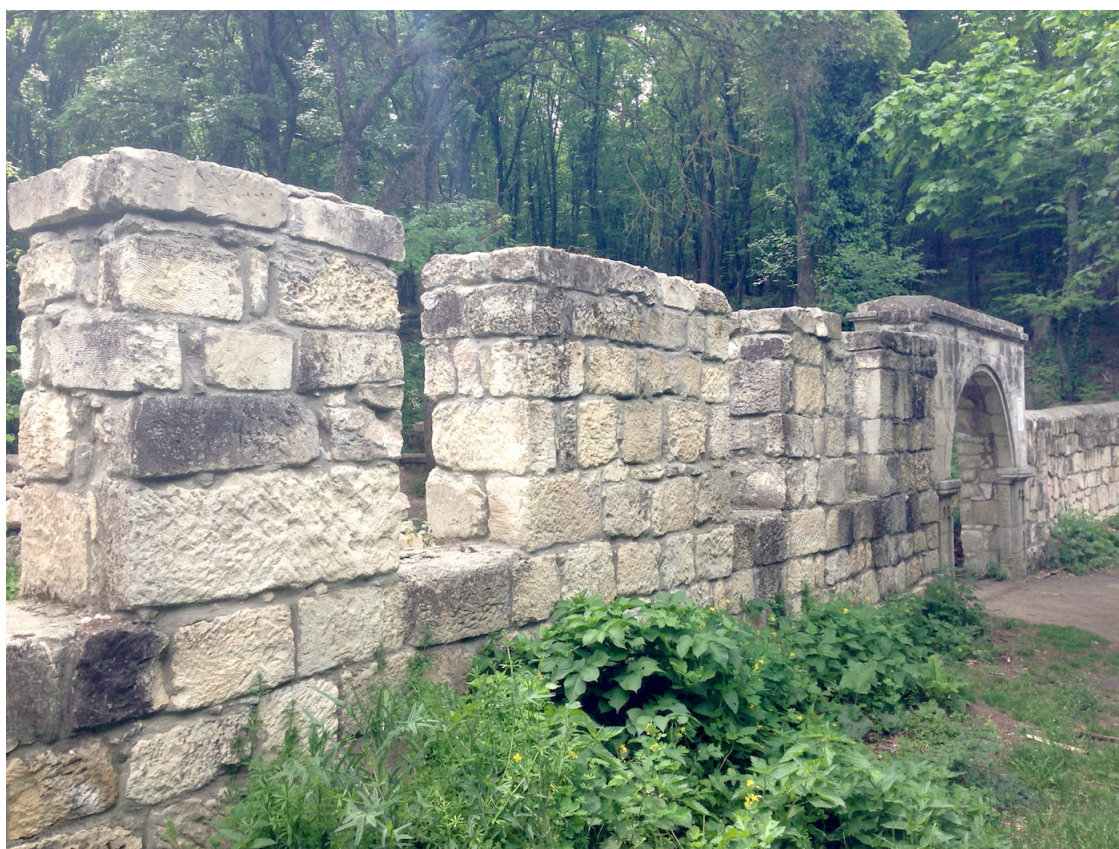
Figure 51. Balta Tıymeş – Entrance gate with the remains of the exterior wall (own photo)
