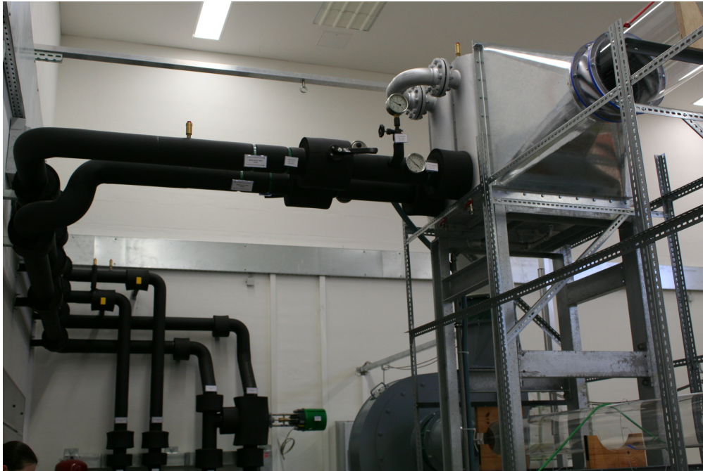
Figure 4.12: Cooling unit with accessories and piping system.
