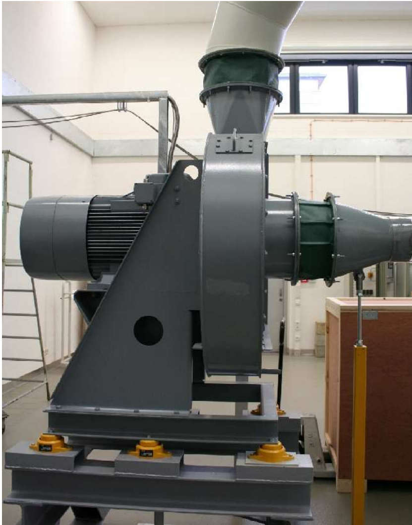
Figure 4.9: Centrifugal blower with motor and blower support equipped with damping elements. Coupling parts between blower and suction side, and blower and return line to avoid transmission of vibrations.
