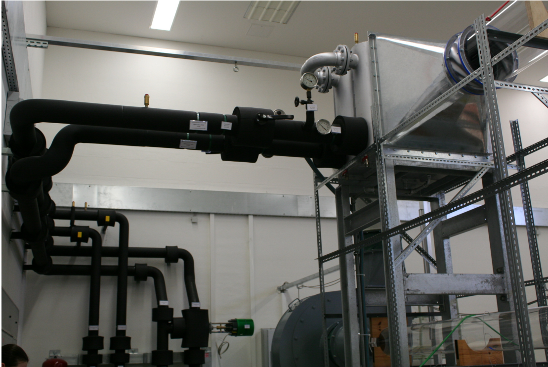
Figure 4.8: Cooling system with heat exchanger (top), piping system (black pipes), pressure control system, valves and accessories.
