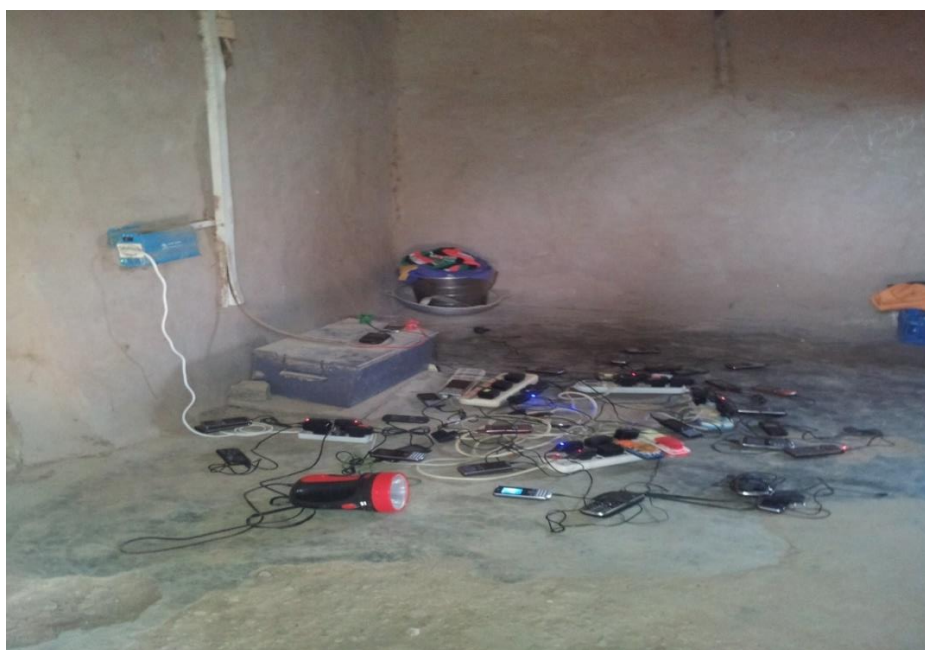
Figure 4-3 Evidence of over-charging gadgets in a community
