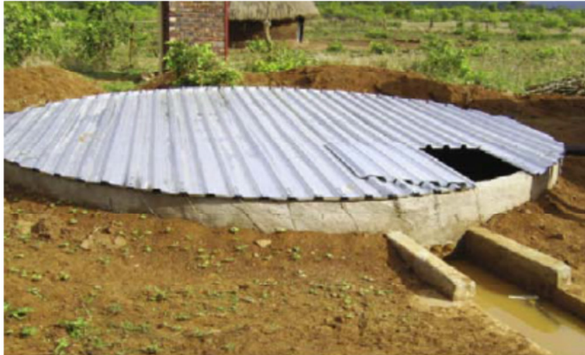
Figure 28: An underground ferro-cement rainwater storage tank.
