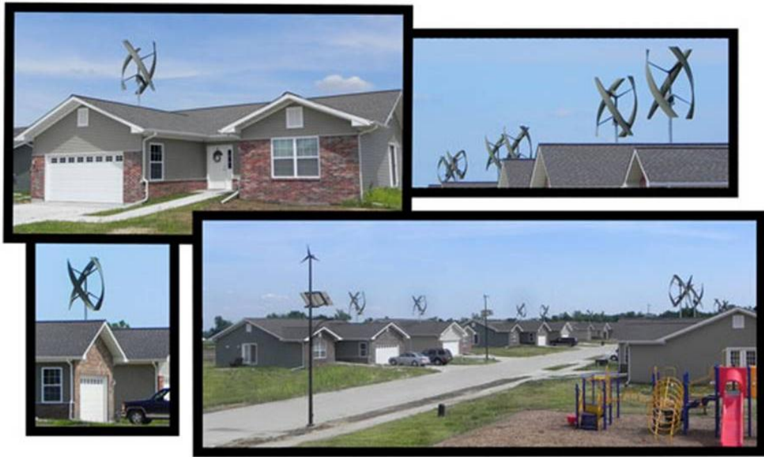
Figure 3.8: Integrated photovoltaics and small wind turbines in Lexington Farms Community in Jerseyville [32]
