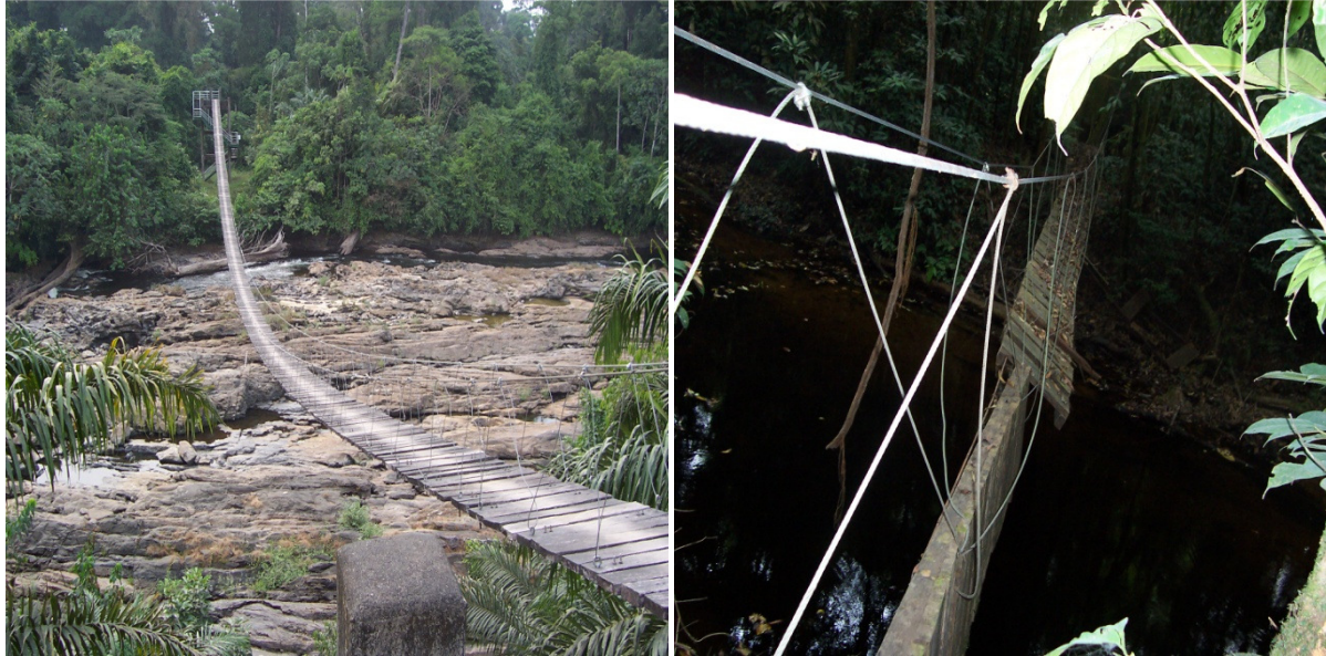
Figure 6. 3 Mana suspension bridge (left) and dilapidated bridge within KNP
