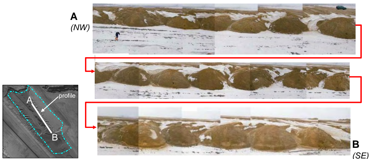
Fig. 27: Longitudinal section across the catchment during the construction phase in March 2005: internal ripple structure.
