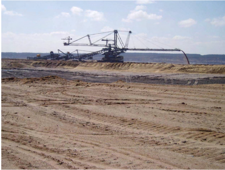
Fig. 8: Technical equipment used in the construction of the artificial catchment: Stacker dumping sandy substrate in Welzow-Süd.
