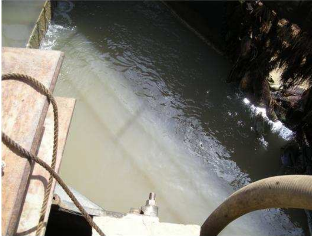
Figure 3.2 Outlet of Treated Waste Water to Receiving River
