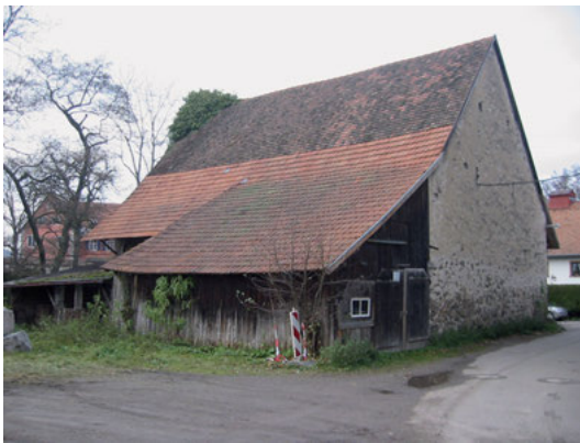
Fig. 2: The barn before its restoration; view from the south. © Sutter KG 3 Kirchzarten.
