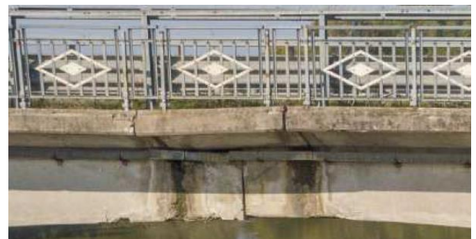
Figure 4 Different heights of the deck at the expansion joint.
