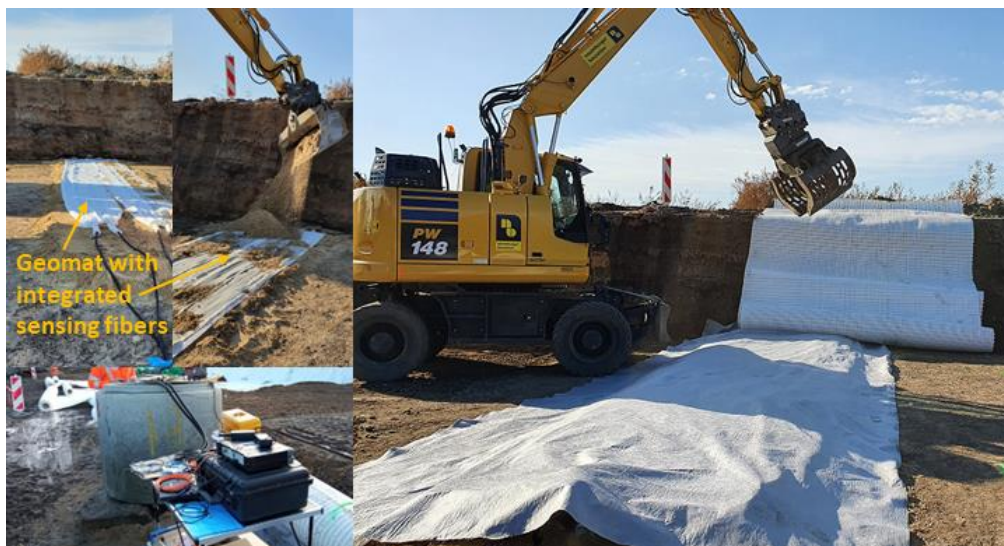
Fig. 6. Installation of sensor-based geogrids under construction site conditions into a road embankment along B91 near Leipzig.
