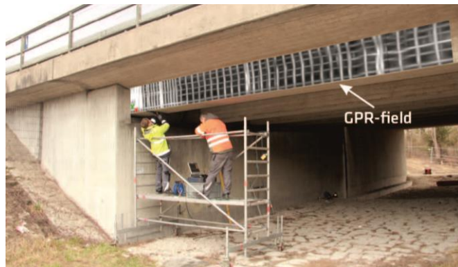
Figure 5 The investigated prestressed concrete bridge with embedded GPR scan indicating the shear stirrups; extracted from [20]
