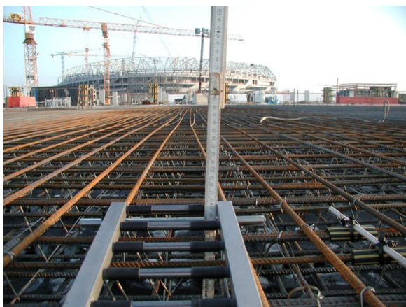
FIGURE 5 Installation of a corrosion sensor “anode ladder” on the upper reinforcement layer. [Color figure can be viewed at wileyonlinelibrary.com ]
