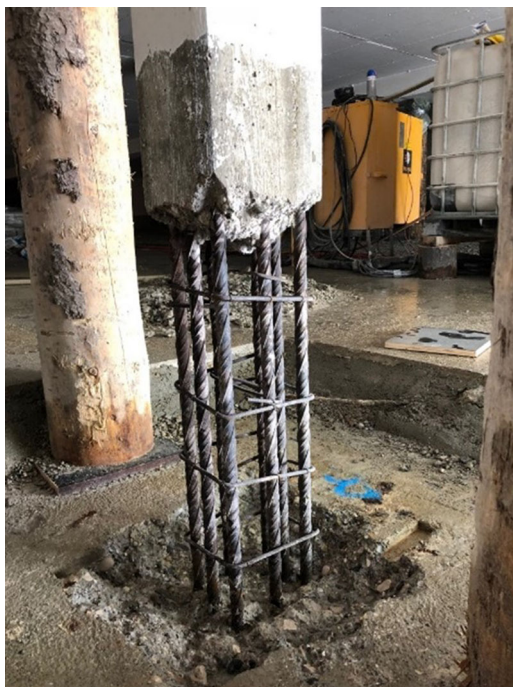
FIGURE 1 Extensive repair of a column in a parking garage due to chloride-induced reinforcement corrosion. [Color figure can be viewed at wileyonlinelibrary.com ]
