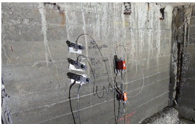
Fig. 6. Different types of AE sensors fixed with magnetic holders inside a box girder.
