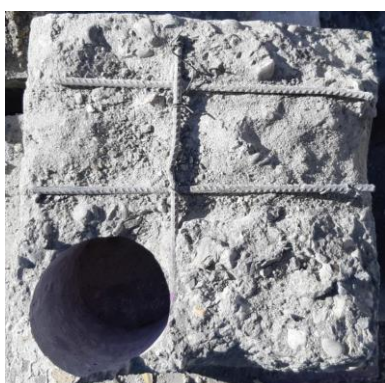
Figure 10 Exposed reinforcement after fire test
