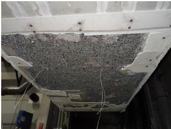
Figure 12 Photograph taken after the specimen was taken out of the furnace day after the fire test (large-scale test)
