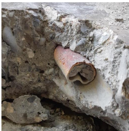
Figure 9 Damaged PVC tube
