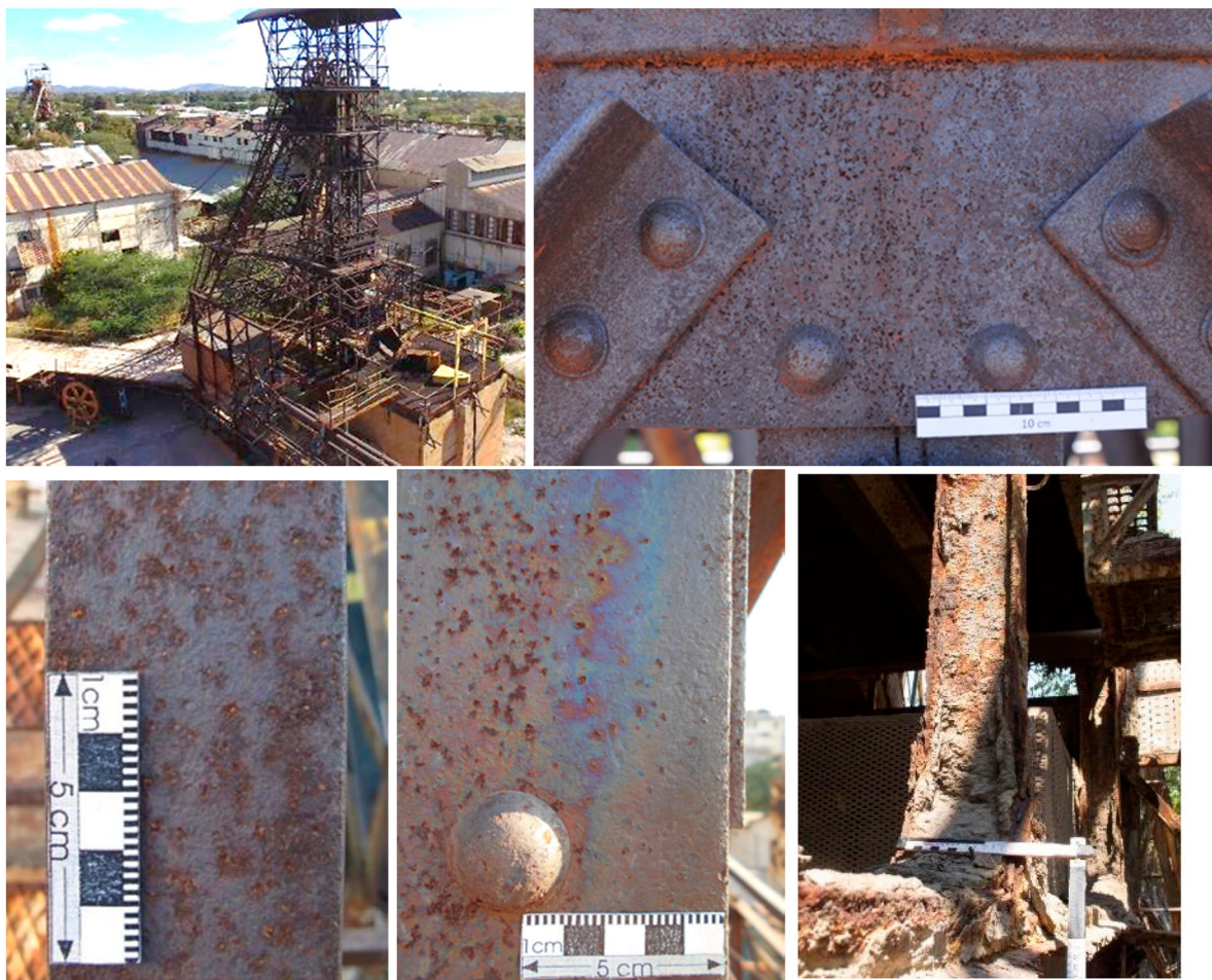
Figure 2. Corrosion phenomena on the steel surface at various regions of the headgear. Upper left: Shaft #1 headgear, overview. Upper right: gusset plate at center main column of Level 2 (south). Lower left: shallow pitting corrosion at a handrail. Lower center: main column at Level 2 (east side) with coating remains. Lower right: ore dust accumulation at the lower column parts.
